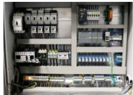
PLC control system (Siemens S7 - 1200)
